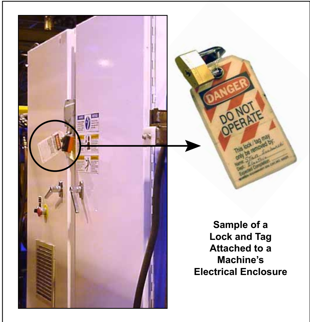
Figure SAFETY-3: Sample of a Lockout/Tagout Mechanism on an Electrical Enclosure
