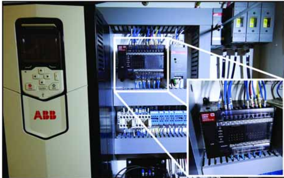
Figure 6-35: Safety Controller, Inside Main Electrical Enclosure
