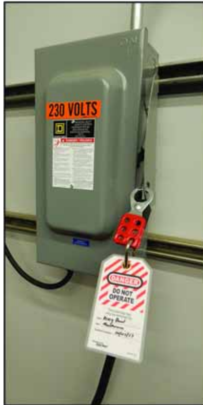
Figure SAFETY-4: Sample of a Lockout/Tagout Mechanism on a Power Source Panel
